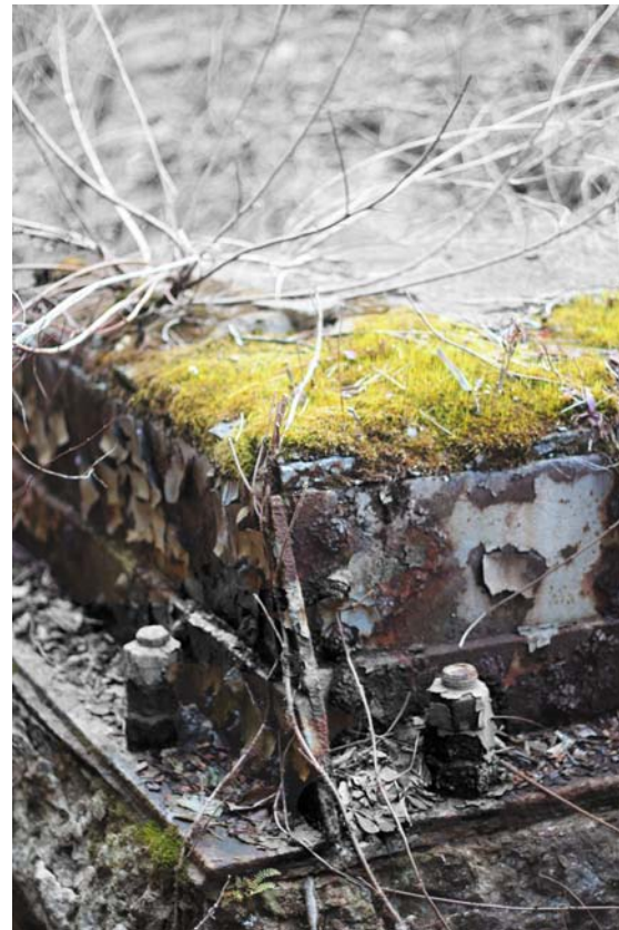
1.1 | Carrie Furnace . Moss Growing on sintering plant
