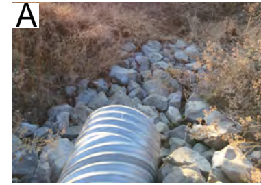
Fig. 4 - 2 Stormwater flow pipe
