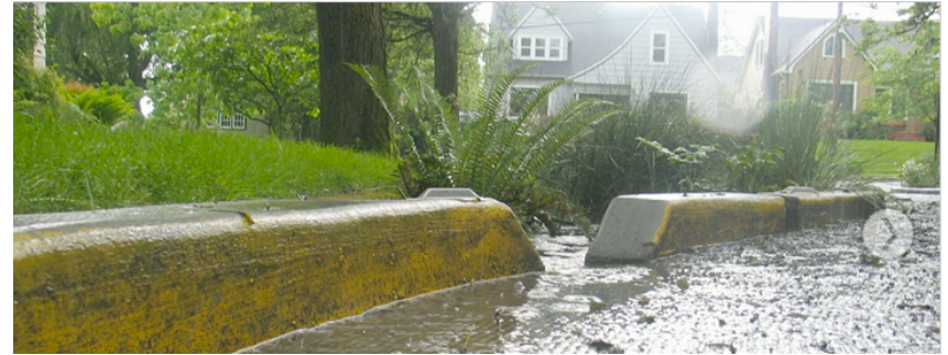
Figure 26 This is a traditional curb cut. It is wide enough to facilitate a significant amount of water and can easily be cleaned if debris collects.
