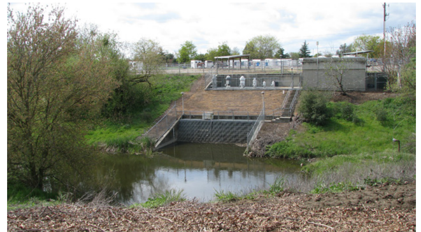
Figure 38. Stormwater Pumps. These pumps are located across the path from the main Arboretum water and pump water to the South fork of Putah Creek. Signage between these two locations could help educate visitors on stormwater practices. (A. Hendrie)
