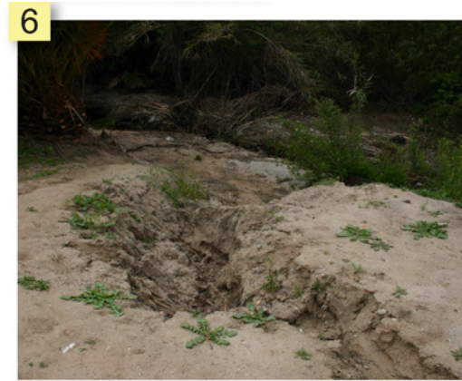
compaction, crevasses from erosion Figure 3.6.
