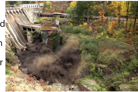
Figure 3.1: Condit Dam Removal. All the water needs is a way of escape. Dave. 2011.
