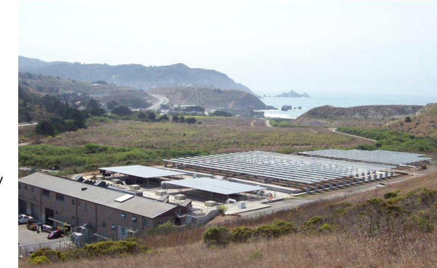
Figure 5.3: Calera Creek Water Recycling Facility . This plant, located in Pacifica just south of San Francisco, offers positive precedents for the bay area. It recycles million of gallons a year while generating a substantial amount of energy. Julie Littman, 2010.
