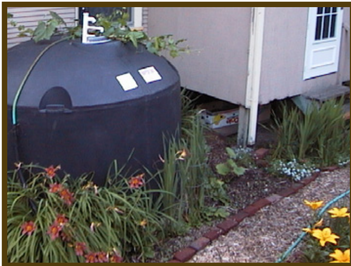
Image 4.6 Rainwater Catchment System
