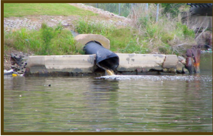
Image 4.1 Point Source Storm Water Drain
