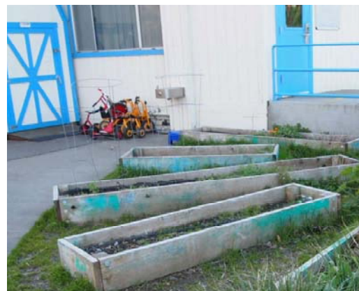
Figure 1.5 Neglected planter boxes
