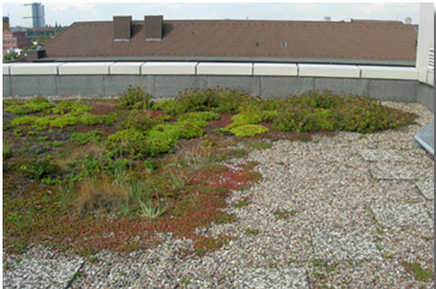
Waterproofing Membrane Protected by a Green Roof System
