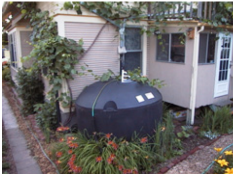
3.2 - Rainwater cistern at home residence in Portland, OR
