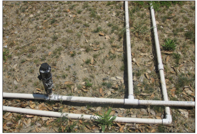
Figure 31: Temporary Irrigation System
