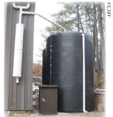
Below: Large storage tank showing first flush device and overflow piping.
