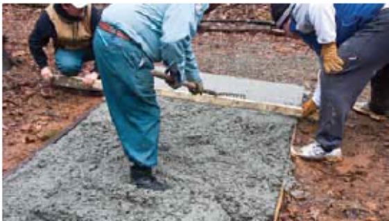
Once enough concrete is in the form, use 2x4 to screed, filling all areas.
