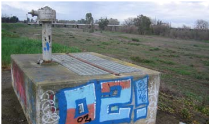
Figure 4.8: The Check Gate valve box
