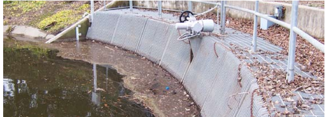
Figure 1.3: Gunk building up in the West end of the waterway.
