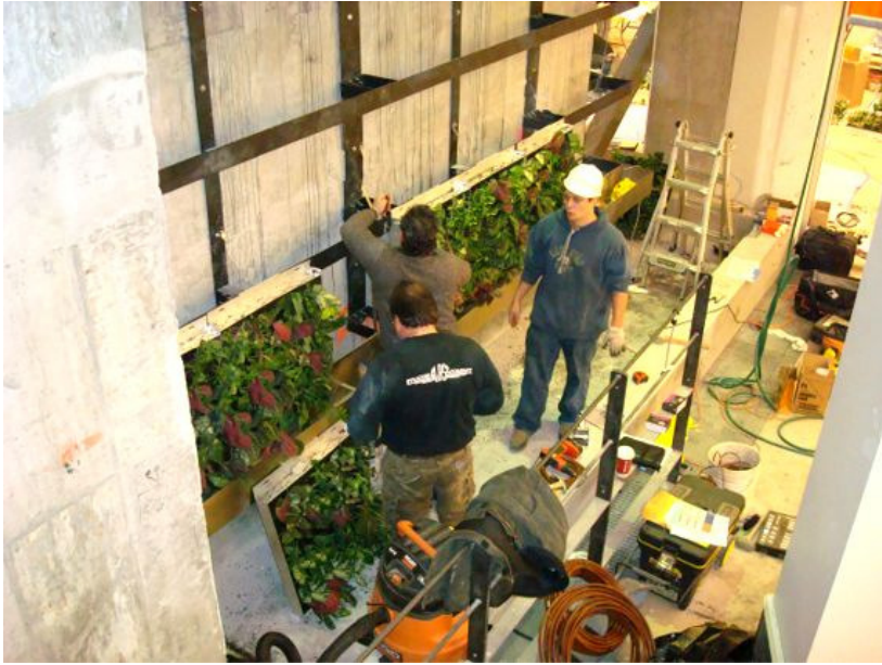
3.2. The exposed mounting frame during construction of a living wall (The Greenroof Project Database, 2006)
