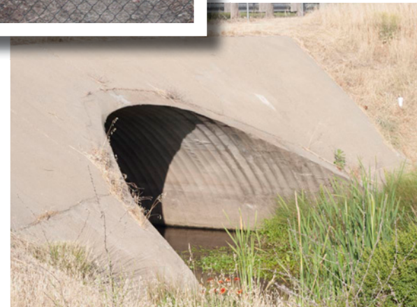
Figure 26: The creek is directed into small pipes to cross beneath roads.
