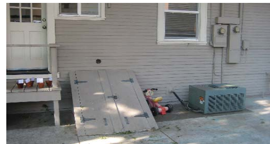
BASEMENT ACCESS DOORS & AC GENERATOR EYE SORES
