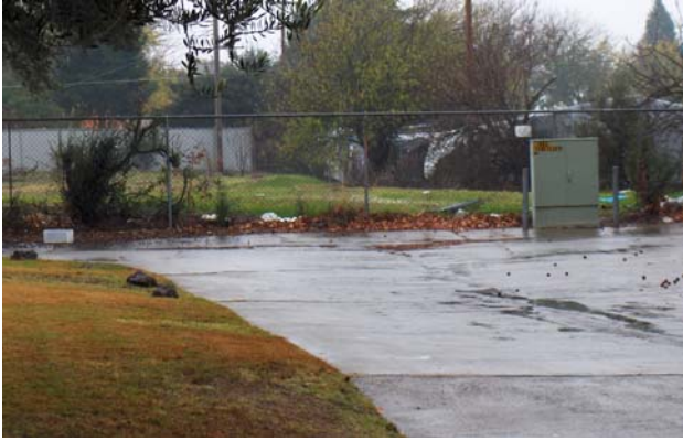
Future connection on the south end
