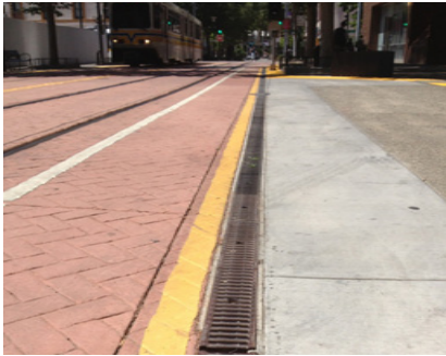
STREET STORM DRAINS
