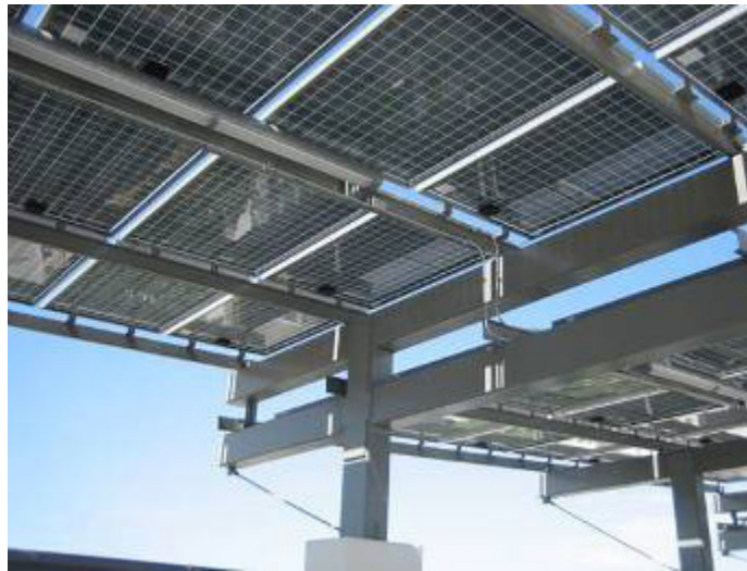
FIGURE 2.48: Solar Panels On Top Of the Parking Structure
