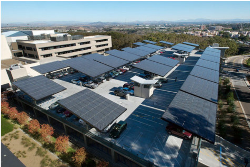
FIGURE 2.46: A Parking garage with photovoltaic panels at the University of California at San Diego
