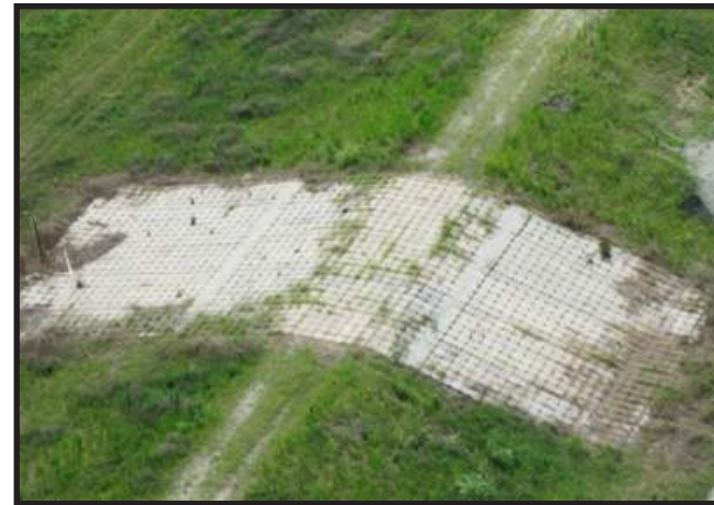
Figure 18. - Aerial photograph of a levee in New Orleans with flood control structure to control erosion. Erosion typically occurs along hard-soft interface. (Source: Berkeley Independent Investigation Team 2007)
