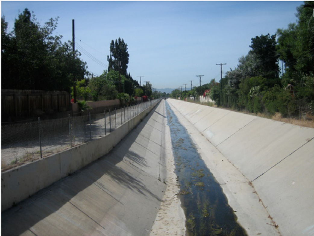
BULL CREEK - BEFORE REHABILITATION
