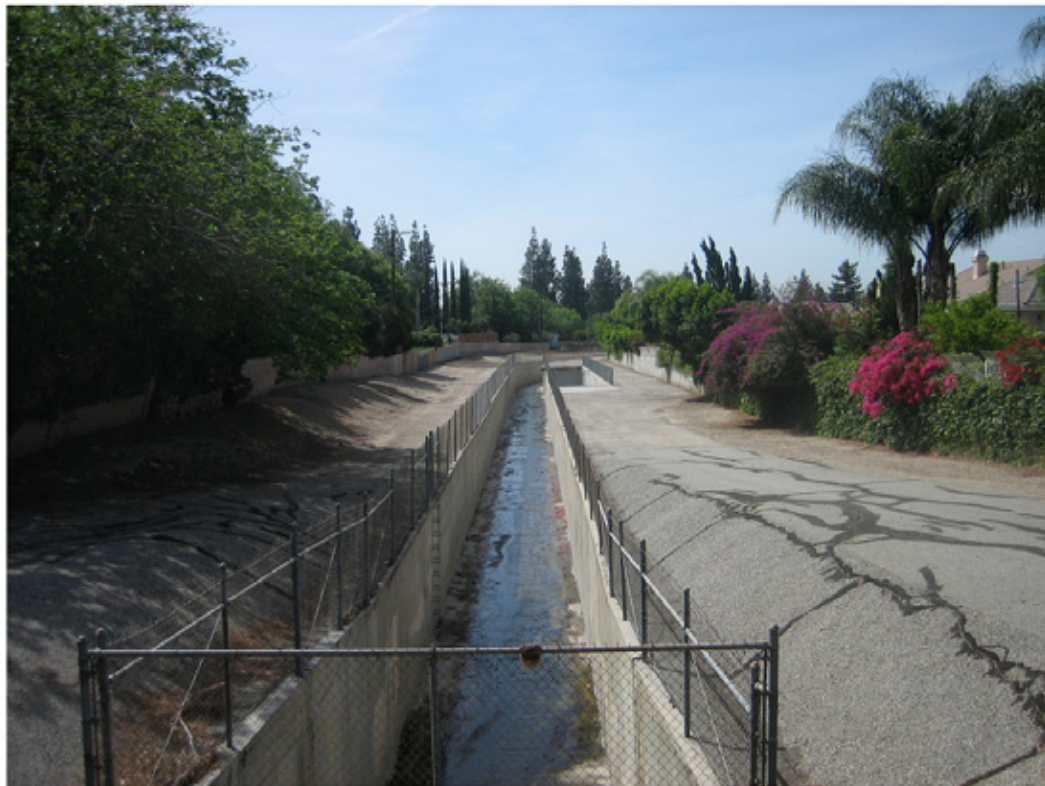
WILBUR WASH - BEFORE REHABILITATION
