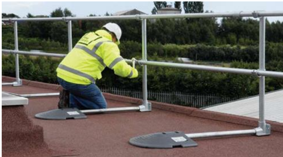
Fig. 5.04: Aluminum railing added to a building for public safety.
