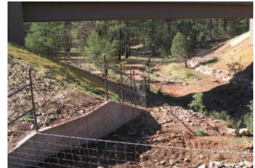
Figure 4-12 Wildlife escape ramp with concrete retaining wall (Arizona Department of Transportation)
