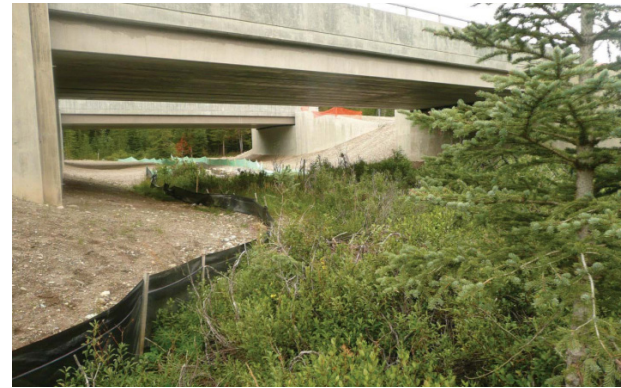
Figure 4-8 Underpass with water flow (Federal Highway Administration, 2011)
