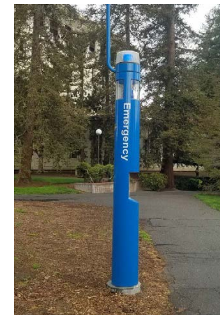
Figure 71 : Emergency button tower in UC Davis. Source: UC Davis Police Twitter
